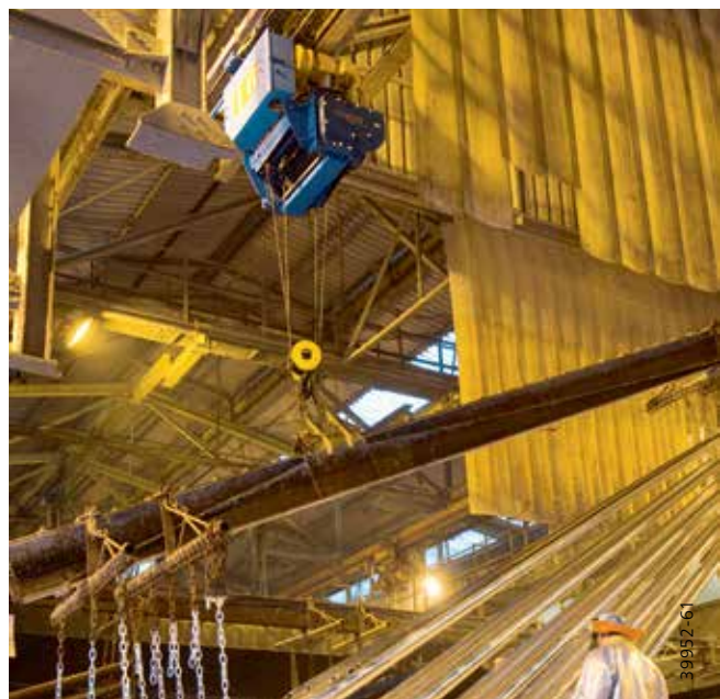
Semi-automatic monorail circuit with rope hoists in tandem operation
